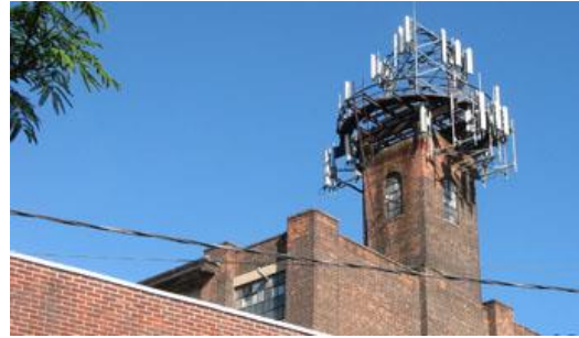
Rooftop cell site
